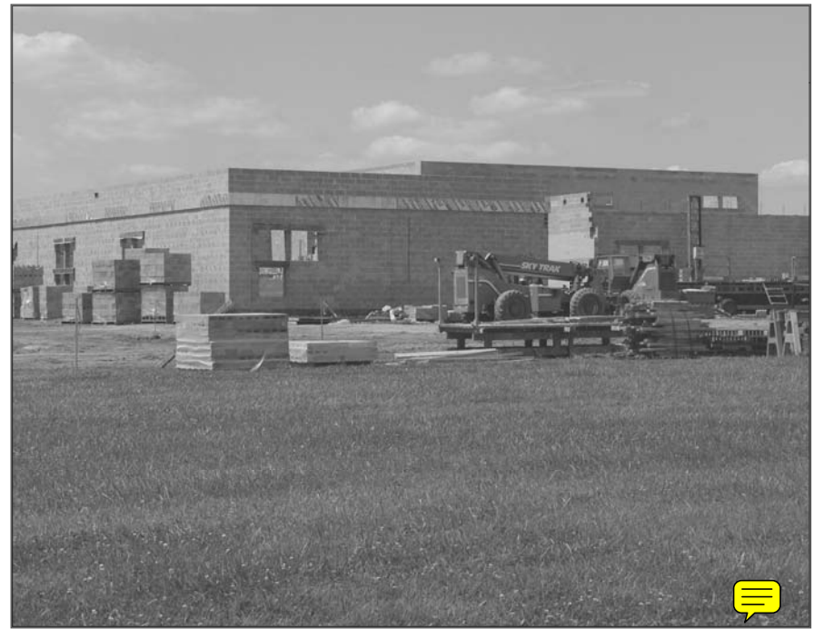
West building is under construction and should be completed by summer of 2009.
